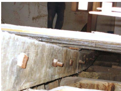
Fig. 14 “Lateral buckling cord compression from one of the main beams”
