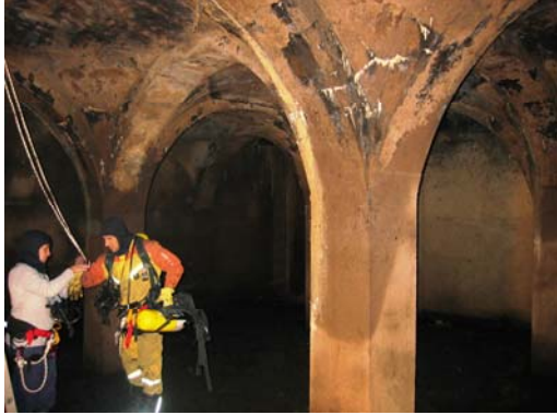
Fig. 5 “Details of the inspection in the underground water tank of the east cloister”
