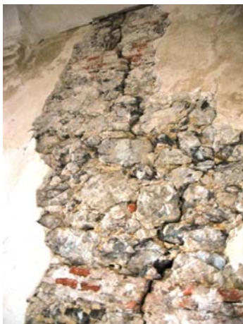
Fig. 16 "Taste and cracking on the west wall of the East staircase. Landing between 2nd and 3rd floor"
